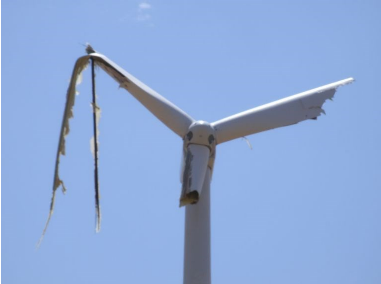
Figure 13: Damaged wind turbine. (Credit: National Oceanic and Atmospheric Administration, no known restrictions on publication.)
