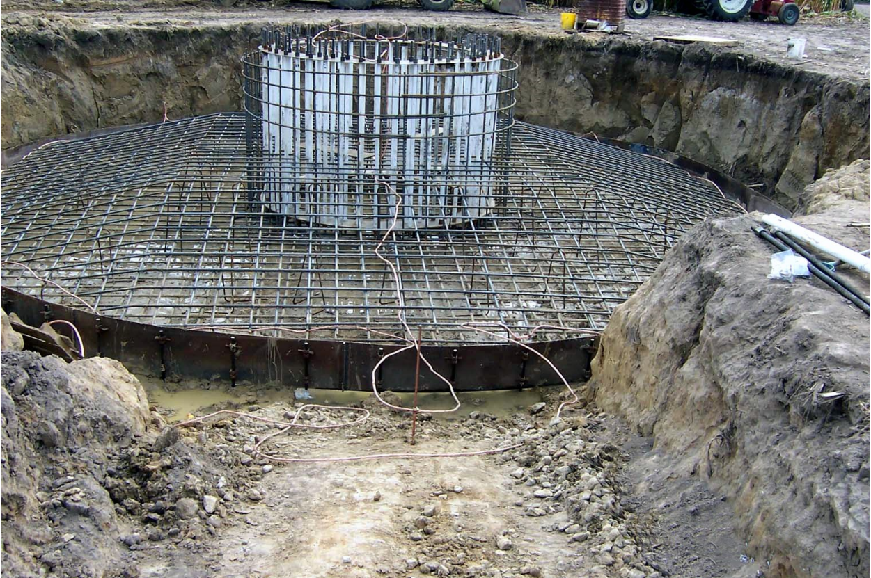
Figure 14: Construction of the base of a smaller wind turbine. Taller and larger turbines would require larger bases. Roughly 6.6 million bases would need to be built and periodically replaced. (Credit: Tradgen Farms, National Renewable Energy Laboratory for the U.S. Department of Energy, used as permitted.)
